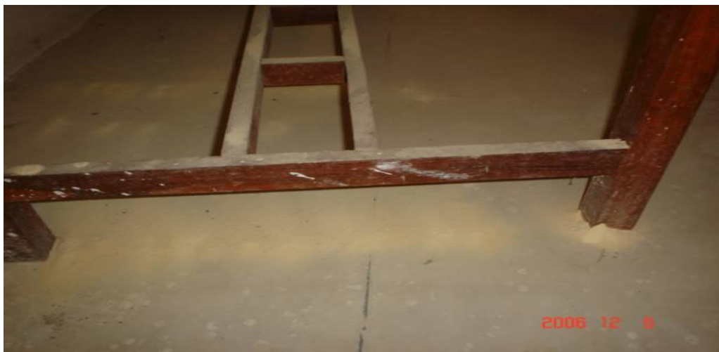
Termites at Work-Degradation of Furniture @ Newly constructed Block of GGHS
