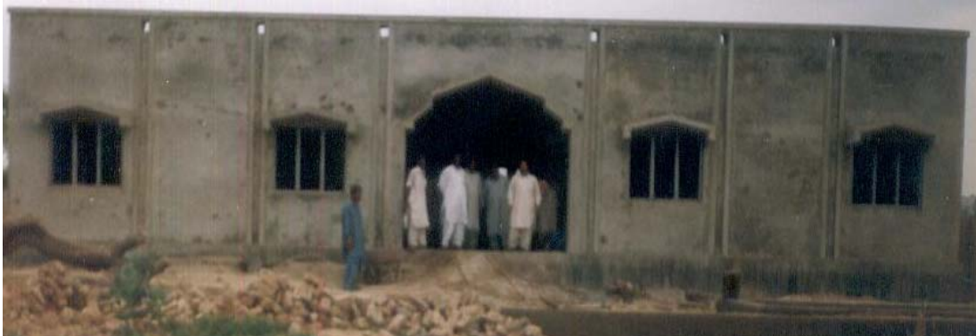
Up gradation of GPS Bhakuo into GMS Bhakuo (under construction) SDSSP ASP 2004-05
