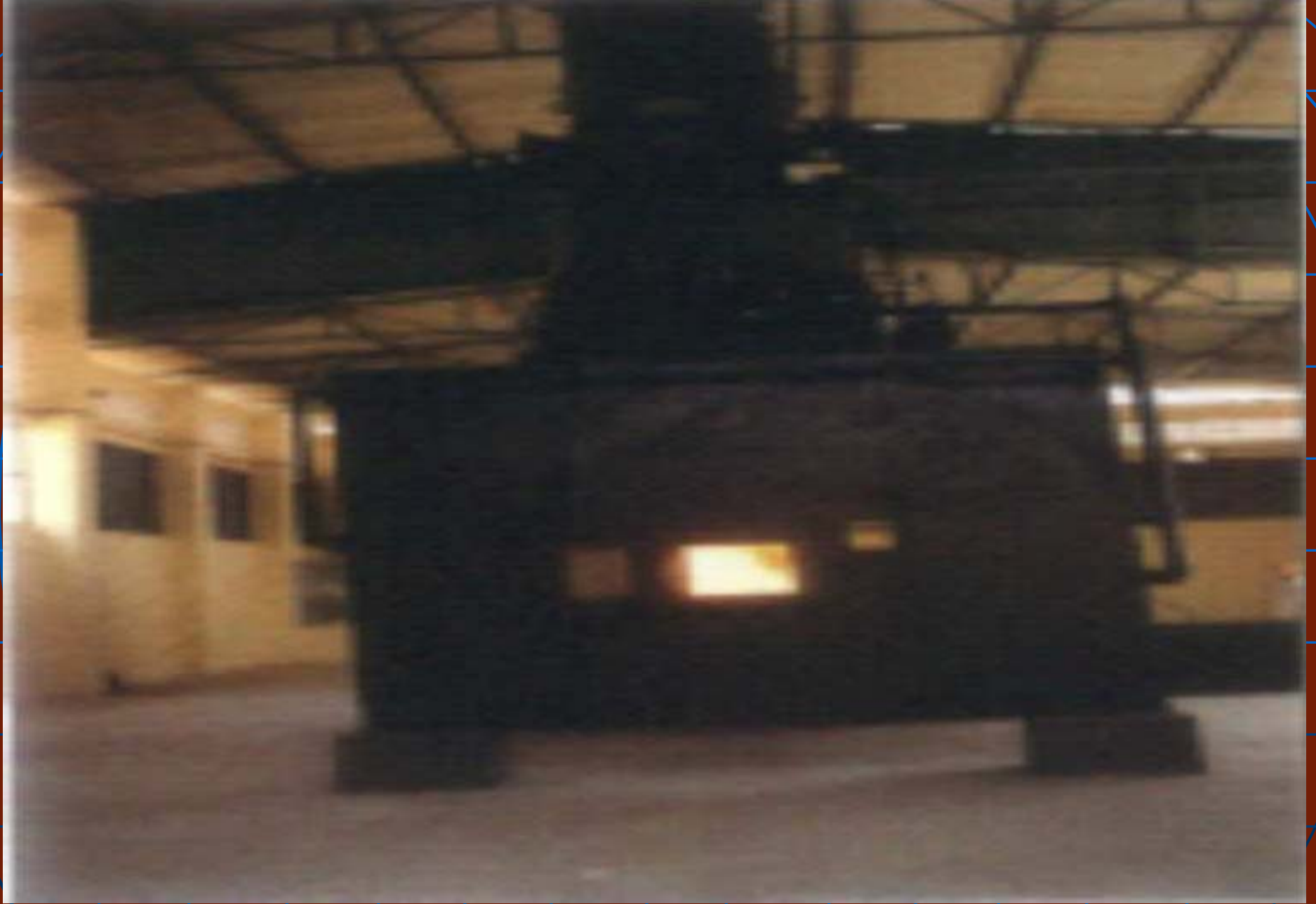
❑ Incinerator Plant at Mewa Shah
